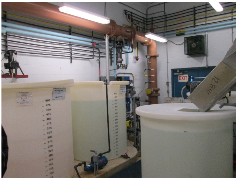
Figure 6.2.2-1 – Chemical storage tanks at the water treatment plant. Two tanks on the left hold the polymer and the tank to the right holds soda ash.
