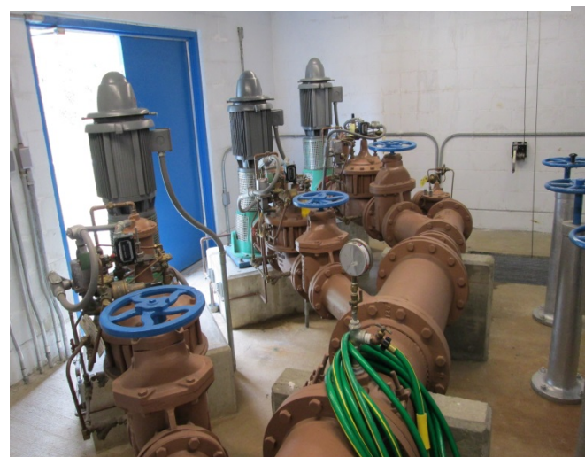
Figure 6.1.3-2 – Three vertical turbine pumps at the intake station
