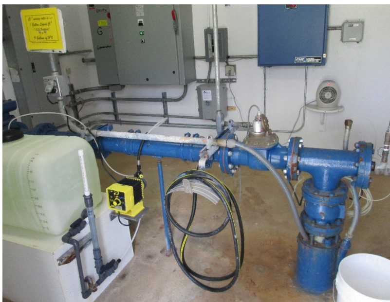
Figure 6.1.4-2 – Inside the Daisy Hill well house. Chlorine injection is shown in the left of the picture.
