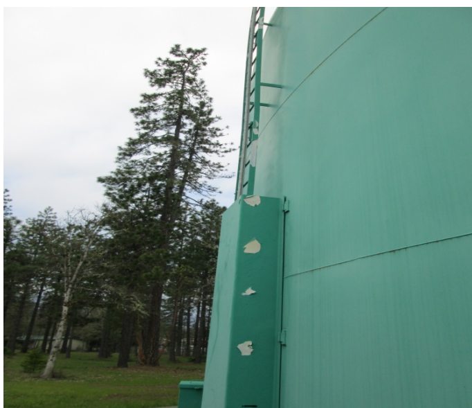
Figure 6.3.2-1 – Clearwell tank at Water Treatment Plant
