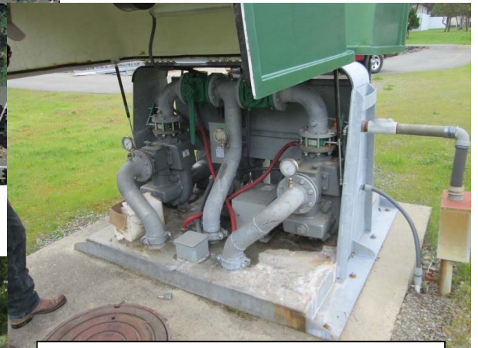
Figure 2.3.4b – WTP PS Pumps and Cover
