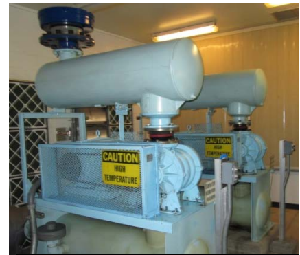
Figure 2.4.4 – Photo of Aeration Blowers
