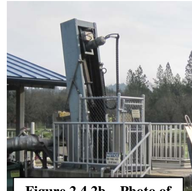
Figure 2.4.2b – Photo of Automatic Screen
