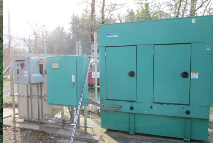
Figure 2.3.2b – North Loop PS Controls and Generator
