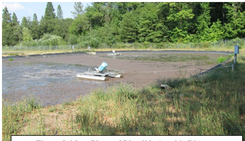
Figure 2.4.9a – Photo of Biosolids Aerobic Digester
