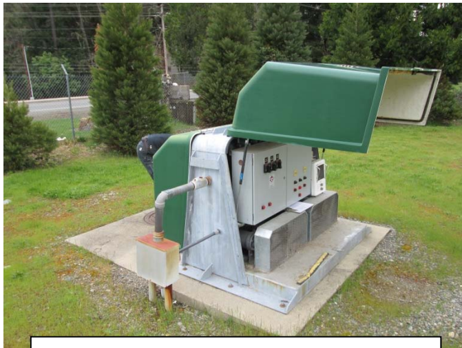
Figure 2.3.4c – WTP PS Controls in Cover
