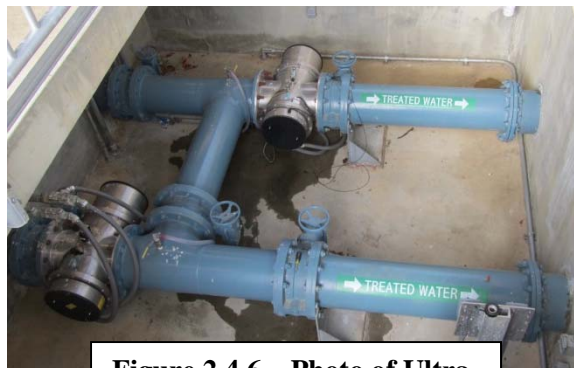
Figure 2.4.6 – Photo of Ultra-Violet Disinfection Units
