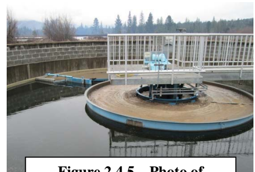
Figure 2.4.5 – Photo of Secondary Clarifier
