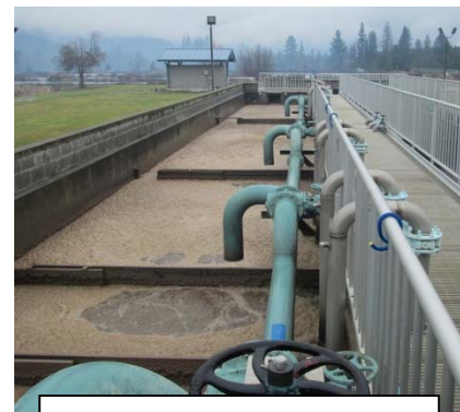
Figure 2.4.3a – Photo of West Aeration Chamber
